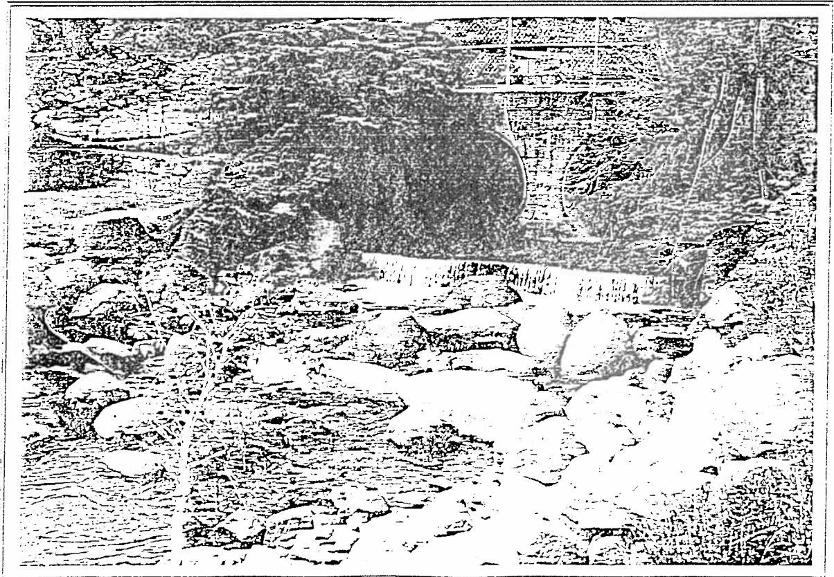
E15. Backwatering of the spillway and installation of a low flow notch could improve fish passage.
