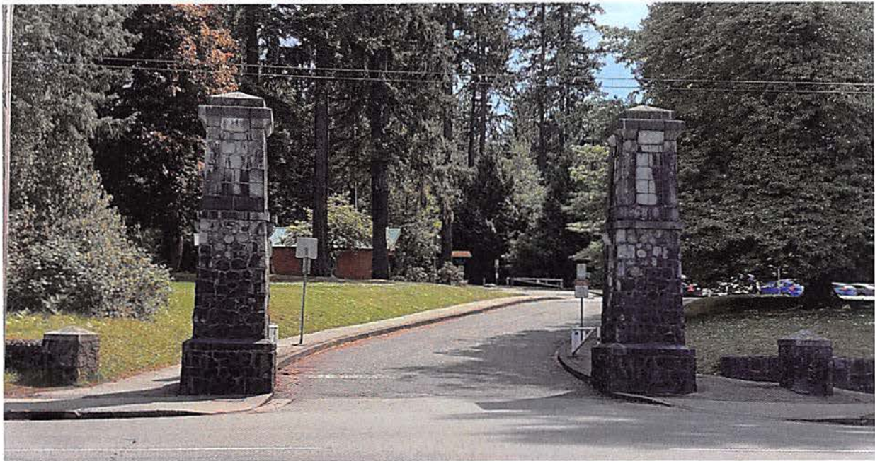
Current condition of the Central Park Entrance Gate pillars
