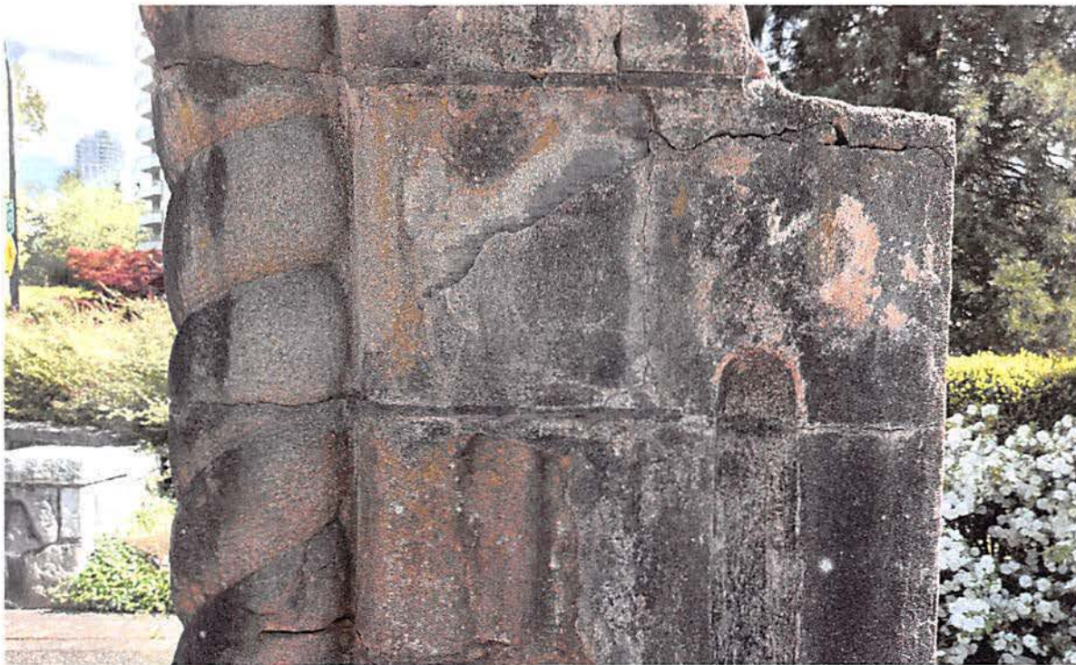
Detail image of area to be repaired through repointing of masonry and stabilization to prevent fractures
